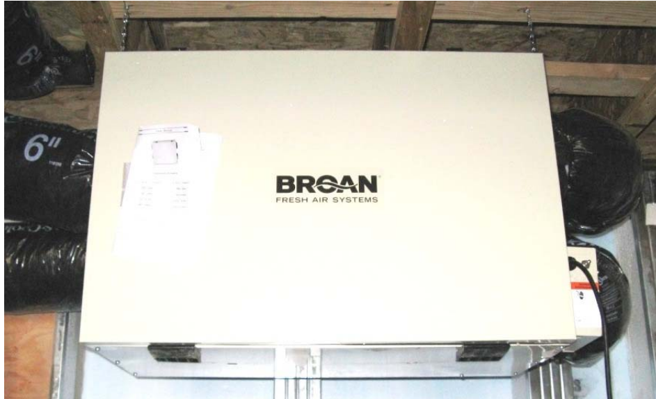
Figure 6. Broan HRV100h for indoor air quality. Note the two 180 degree bends in the supply and return ducts on the right hand side.
